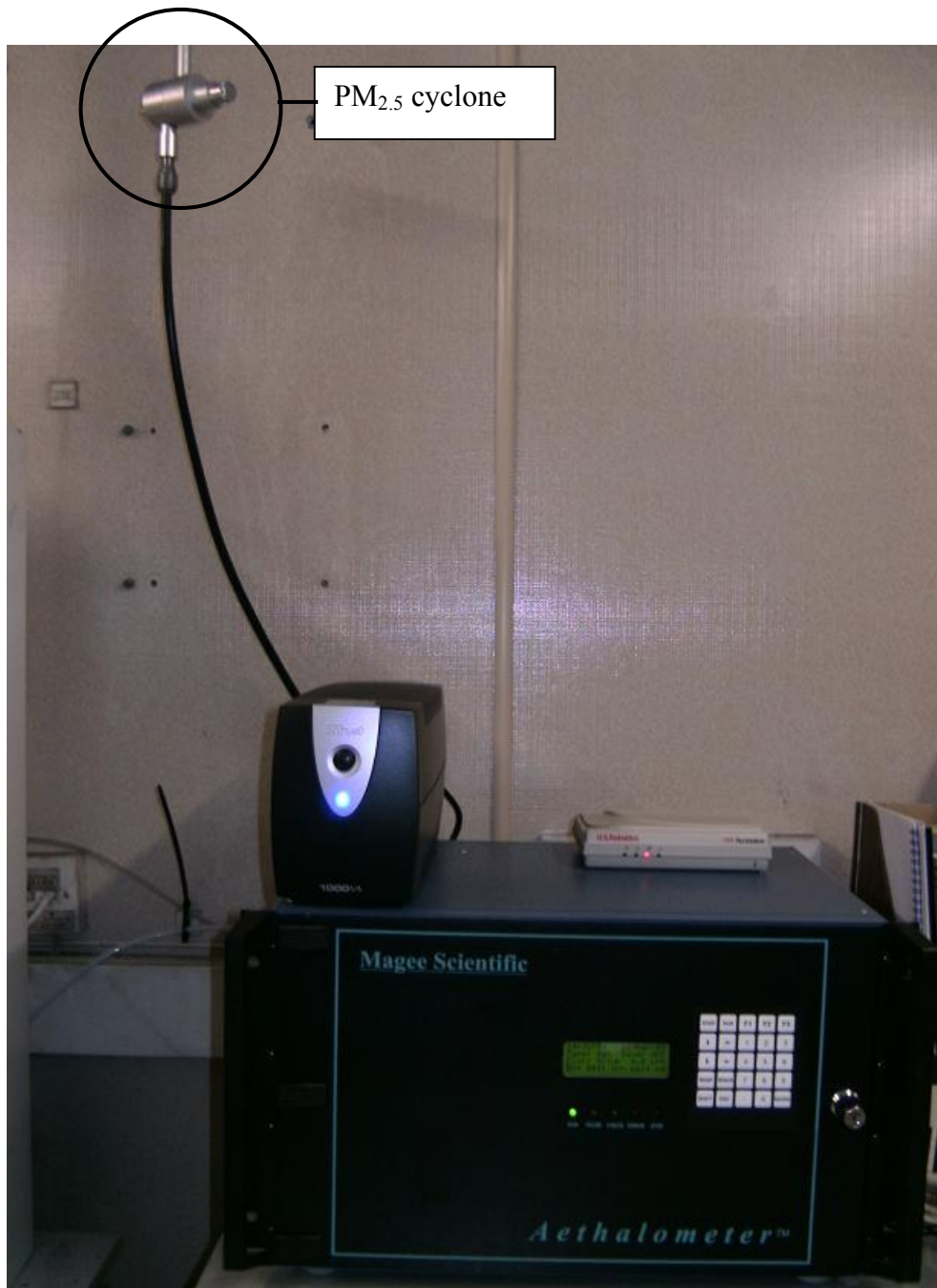
Figure 3a Installation Of Aethalometer And PM 2.5 Cyclone At A Network Site
