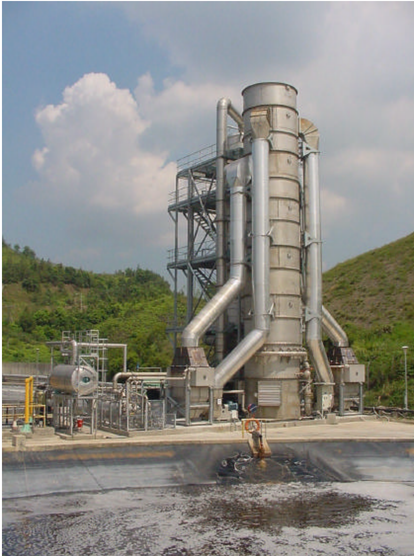
Figure 15. Ammonia burner, using landfill gas to combust the ammonia. Source: Organics (landfill technology company) – Personal Communication
